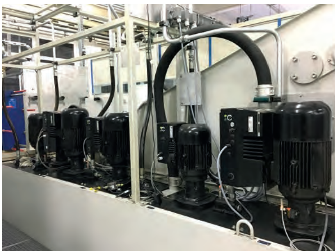
Conventional coolant pumps equipped with air-cooled motors on a filter system
